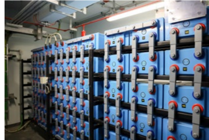
Renewable Energy Storage
