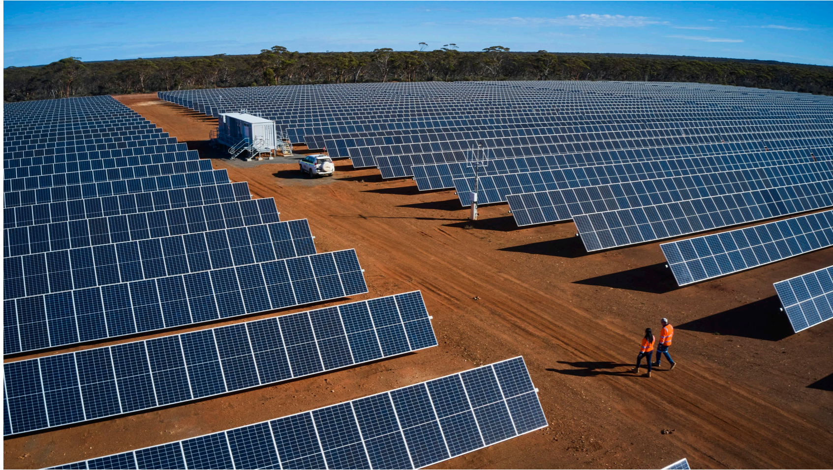
Nova 5.4MW Solar Farm
