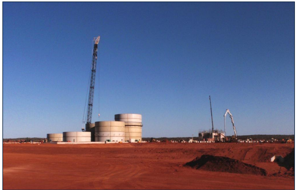
Photo 3: Tropicana Gold Project – CIL Tanks (left) and Ball Mill (right).
