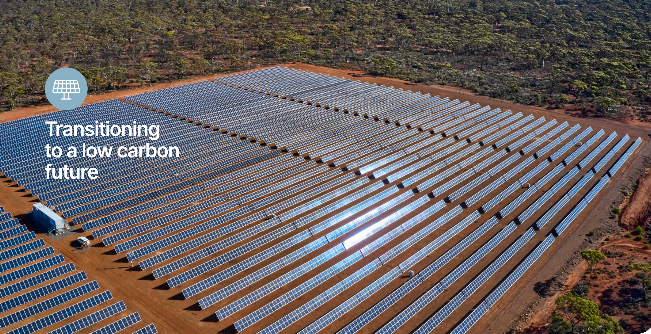
Image: Nova Operation solar farm
