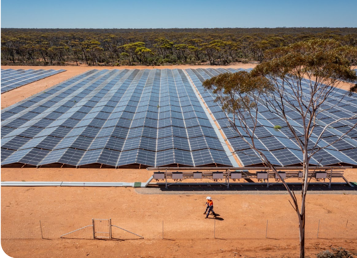
Image: Nova Operation solar farm
